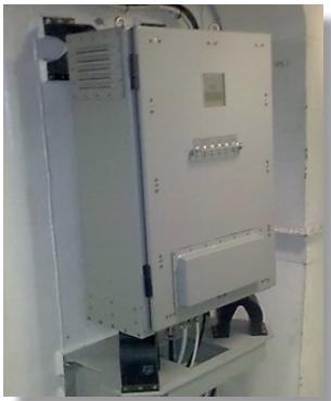
Variable Speed Drive
